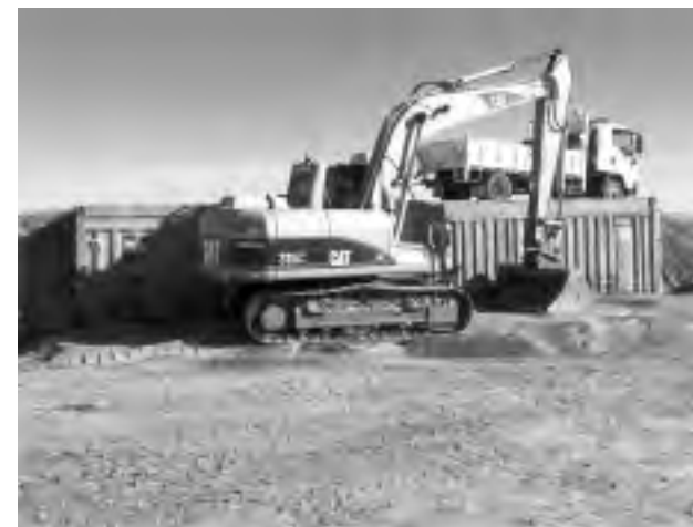
Recycling Transfer Station at Donald Landfill.
